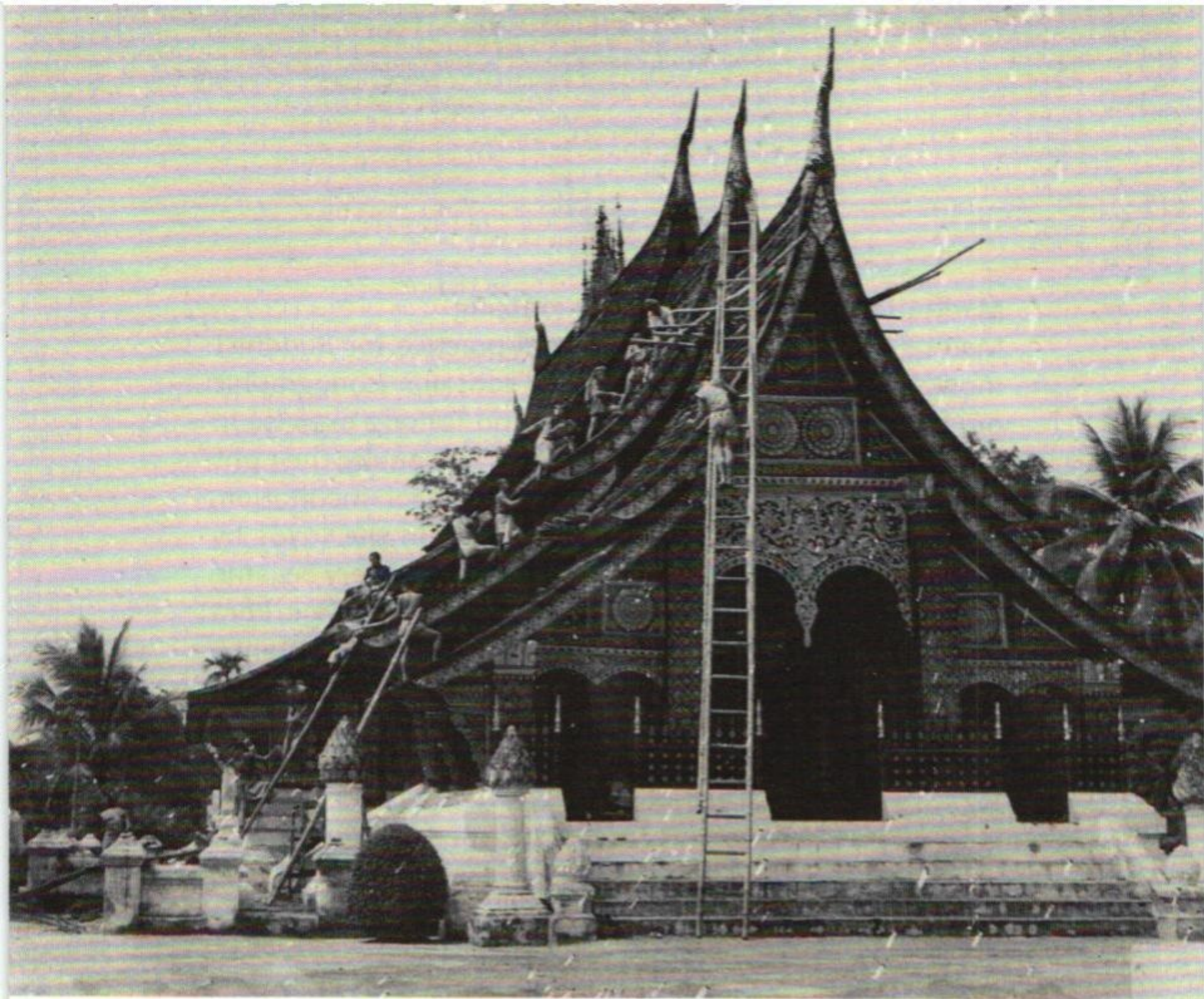
Monks and novices repairing the roof of the Sim of Vat Xiengthong Rajavoravihan. Date uncertain, probably late 1970s
